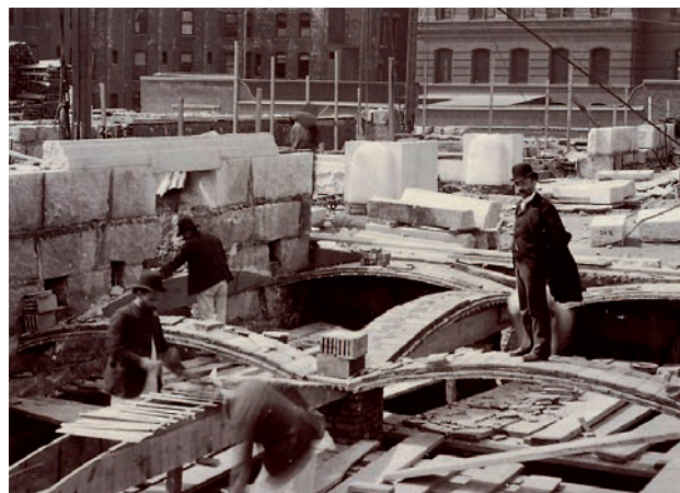
Fig. 3. Guastavino standing up on a newly built arch during the construction of the Boston Public Library, 1889. (Image courtesy of Boston Public Library, “Boylston Street” August 31, 2006 via Flickr, Creative Commons Attribution).
